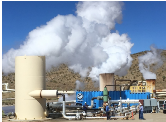
Figure 4. GreenFire Energy's 2019 Demonstration Project at the Coso Geothermal Power Plant, Coso, California
