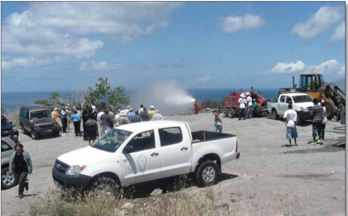
Crews view the N-3 well – a 2,900 ft. slimhole on Nevis. PHOTO BY MAKEDA WARNER.
